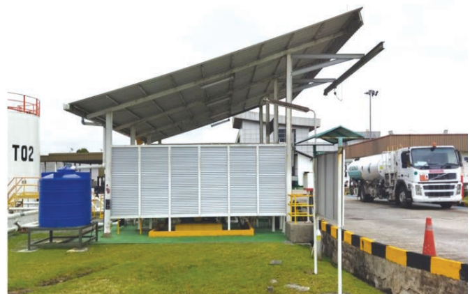
Rainwater harvesting with solar powered pumps at Kuching Aviation Terminal
